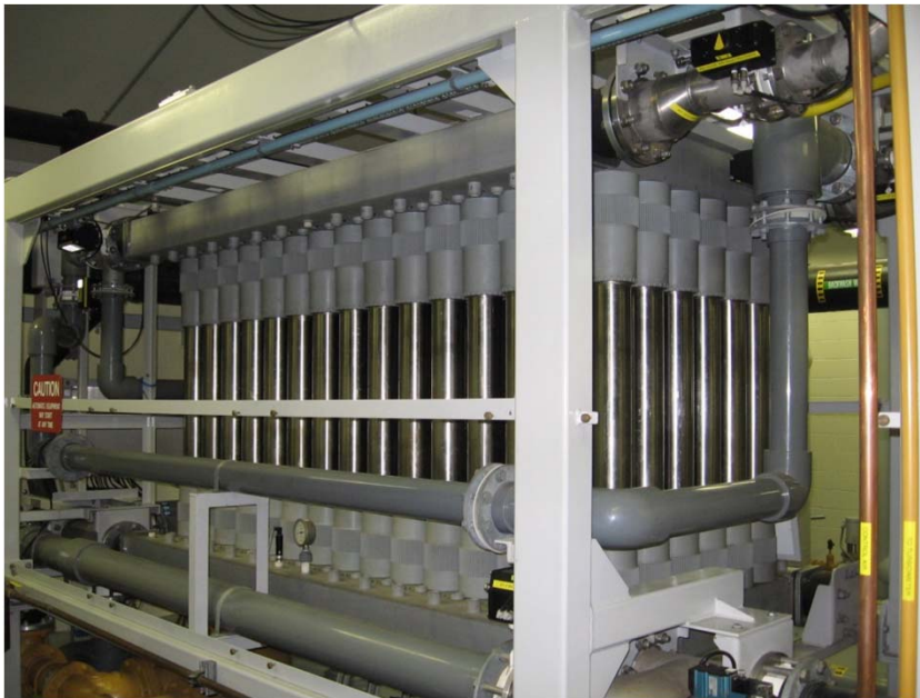
Main Treatment Skid
