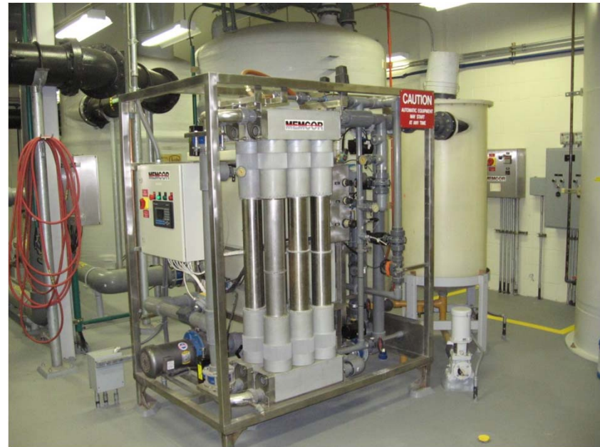
Backwash Treatment Skid
